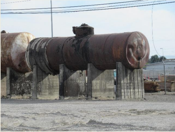
An old tank car on a stand to store some type of liquid
