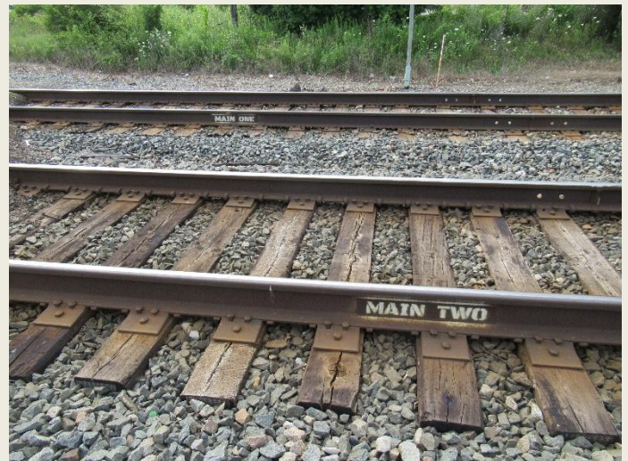
trackage signs - main 1 and main 2 for CN tracks markings
